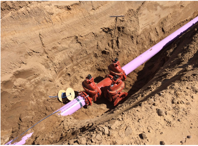
Recycled water main pipeline intersection and restrained valve installation for The Dunes at Monterey Bay Phase 1C project.
