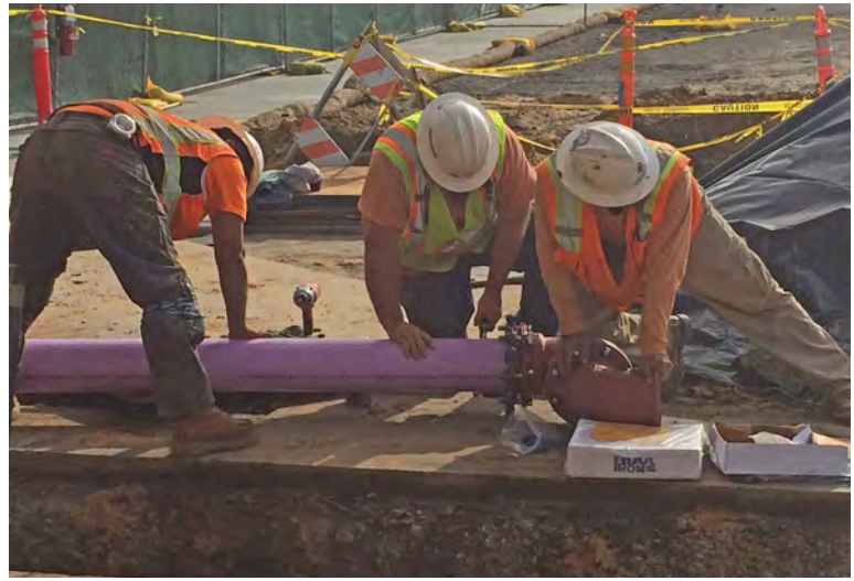
Recycled water pipeline and restrained fitting installation in existing campus roadway for the CSUMB A3 project.
