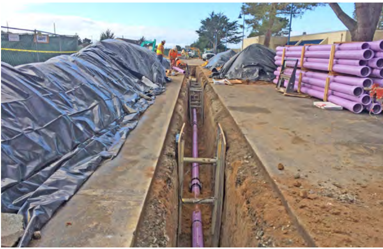
Recycled water pipeline and restrained fitting installation in existing campus roadway for the CSUMB Academic Building 3 (A3) project.
