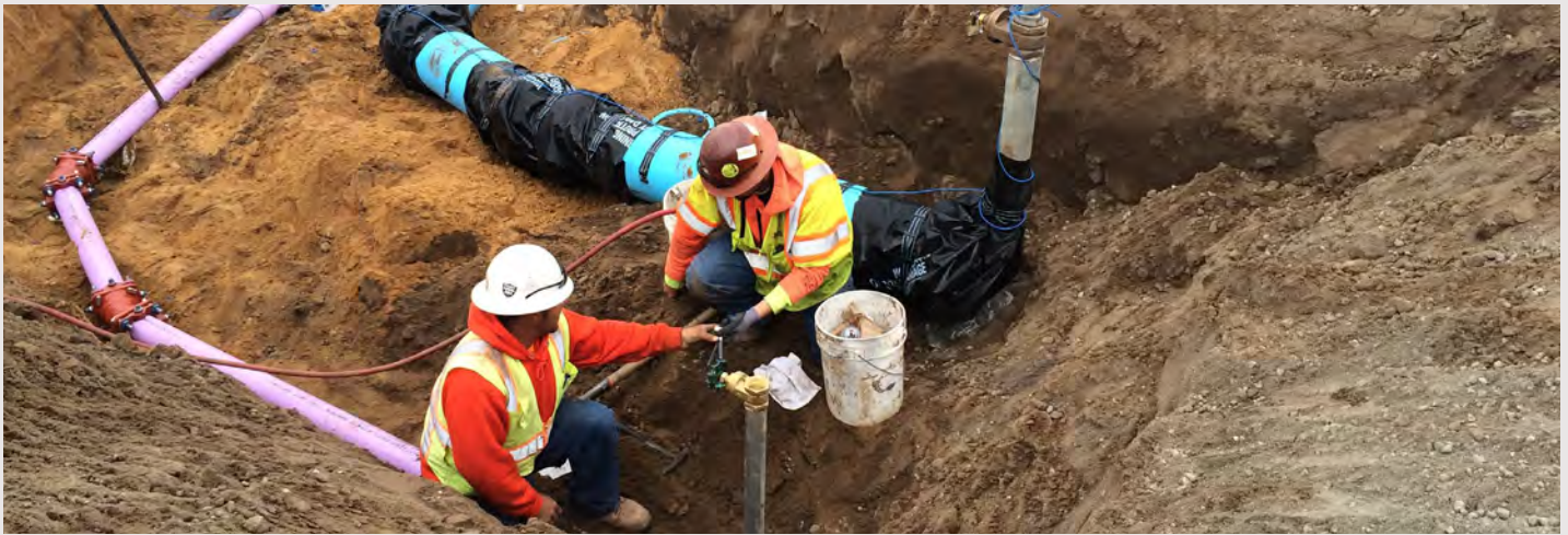
Installation of parallel domestic water and recycled water main pipelines for commercial improvements on The Dunes at Monterey Bay Phase 1B.
